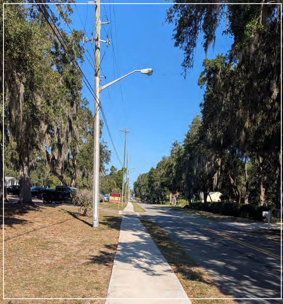
Lighting along the sidewalk on Citrona Drive. Source: Project Team.
