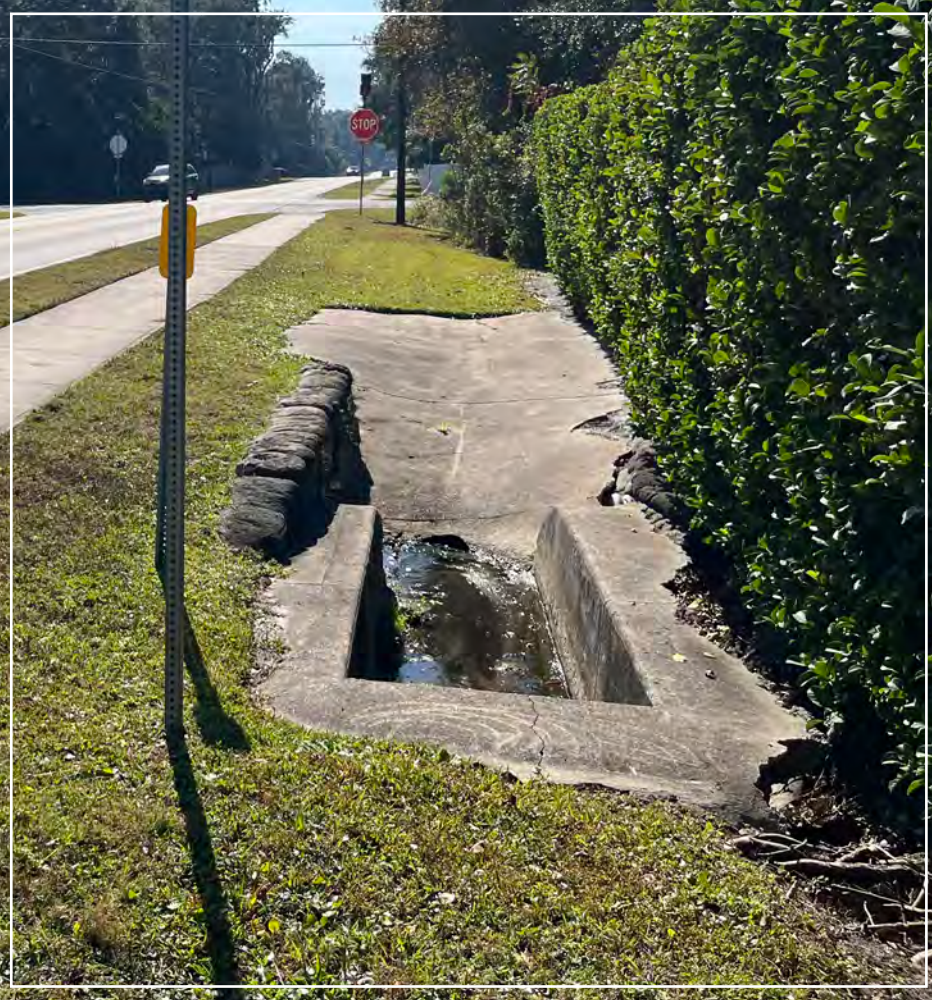
Drainage along Citrona Drive. Source: Project Team.
