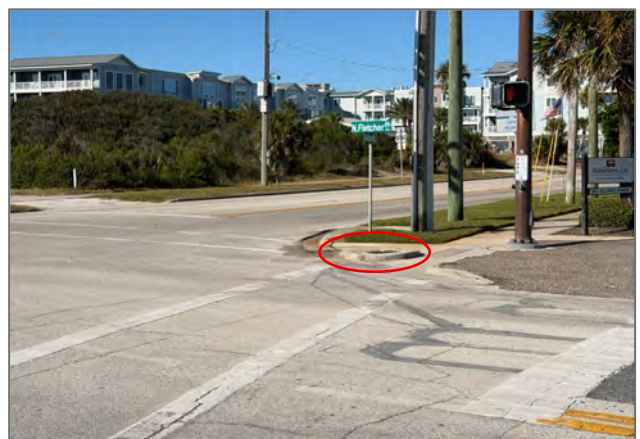
Raised concrete collar protecting sewer manhole at the sidewalk curb ramp on the northwest corner.
