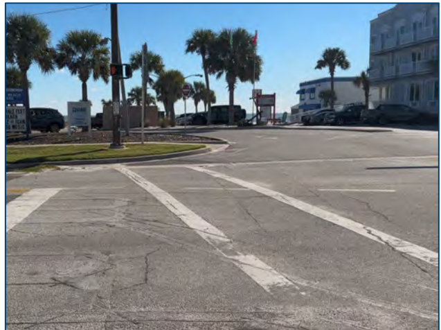
Northeast crosswalk curb ramp is misaligned from the crosswalk location
