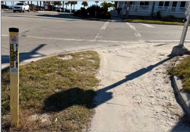
Loose sand accumulated on sidewalk and ramp, creating slip hazard for pedestrians.
