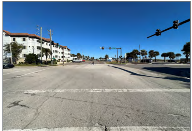
Poor pavement conditions at the intersection of Atlantic Avenue and S Fletcher Avenue, looking northbound
